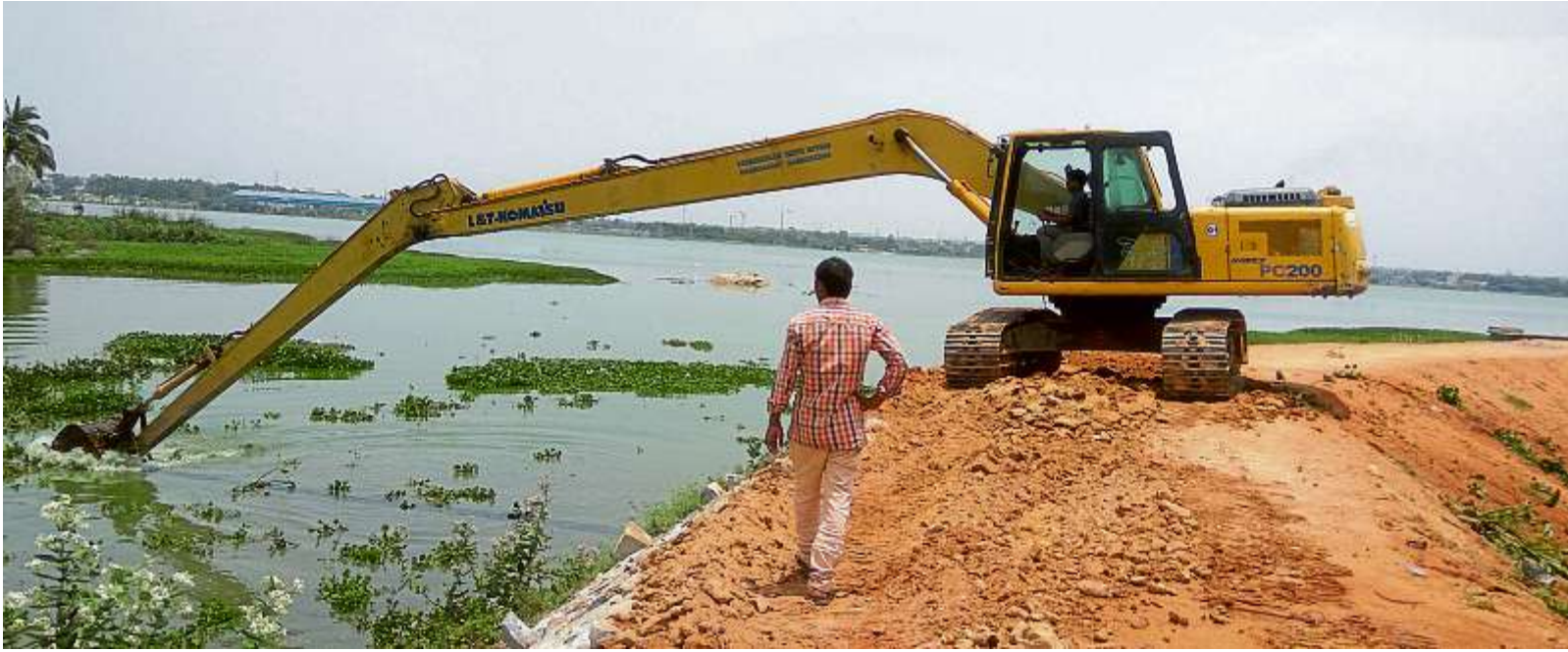
Water in Lakshmisagar Lake at Narasapura in Kolar taluk has already turned green. An excavator removes hyacinth from the water on Friday. DH PHOTO/CHIRANJEEVI KULKARNI
